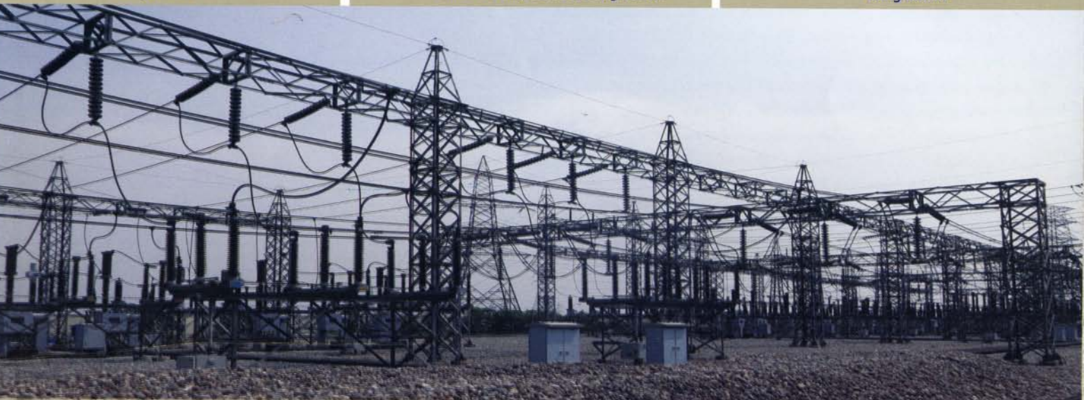
Substation at Aminbazar, Dhaka, Bangladesh
