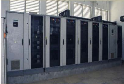
Substation Control Room, Hi-Tech Park, Jessore, Bangladesh
